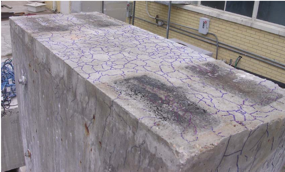
Figure A.31: Map Cracking at Top of Column A
