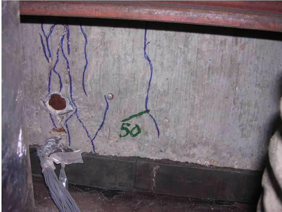
Figure 7.85: Initial Cracking of Post-tensioned #2 Specimen
