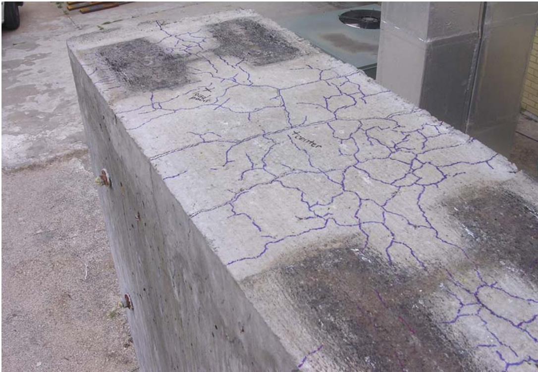
Figure A.32: Map Cracking at Top of Column B
