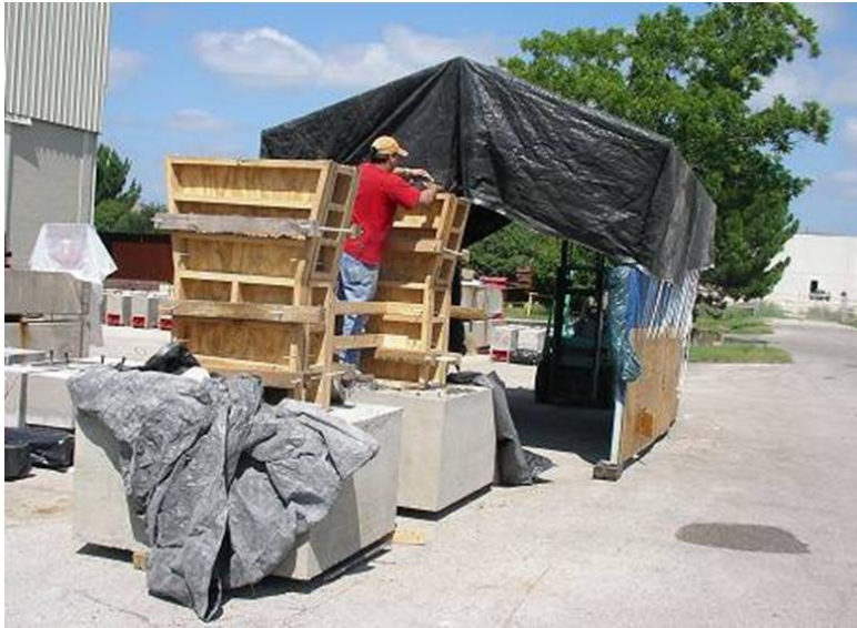
Figure 3.8: ASR/DEF Columns about to Receive Cover 96
