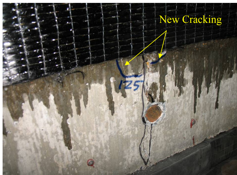
Figure 7.55: Initial Damage of FRP #1 Specimen
