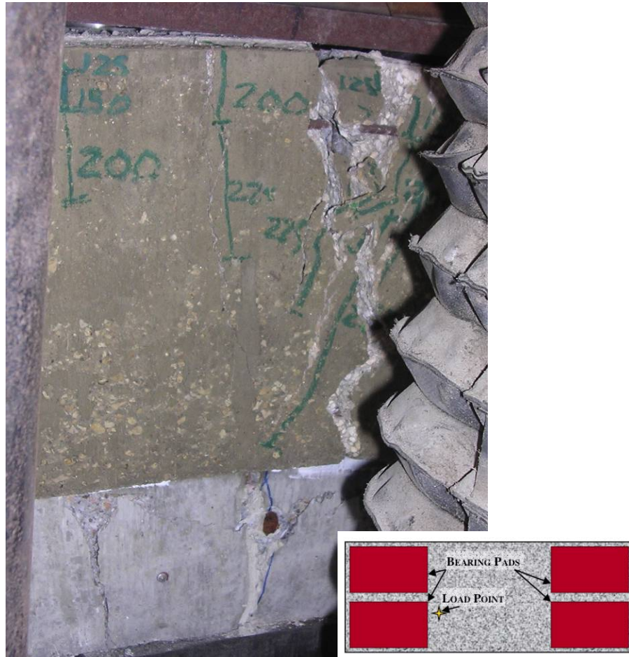
Figure 7.110: Fractured Repair of Concrete Jacket #2 Specimen
