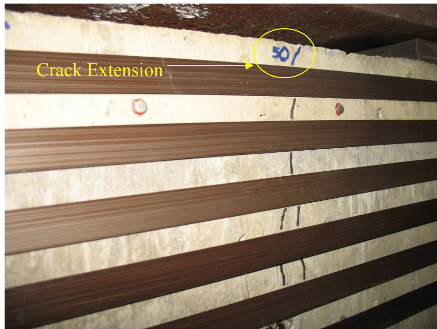
Figure 7.41: First New Cracks on Packing Strap #2 Specimen
