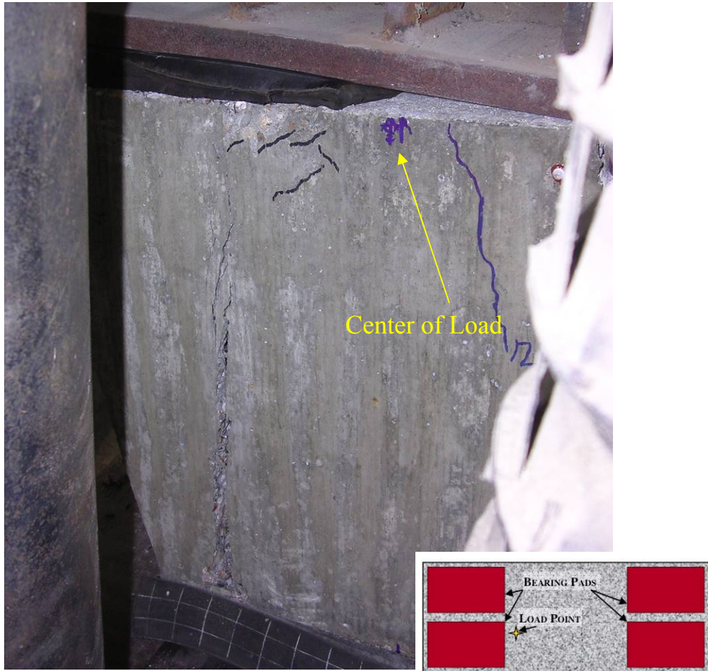
Figure 7.26: Crushing under Heavily Loaded Bearing Pad of Cracked Control
