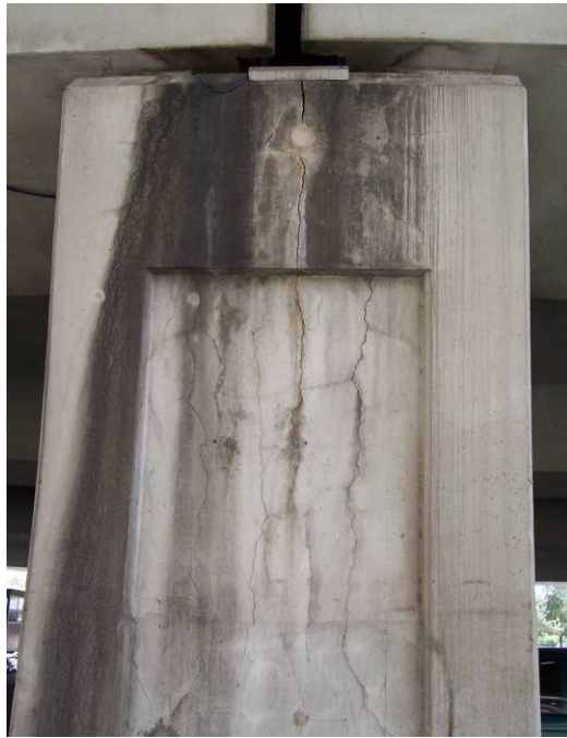
Figure 2.2: DEF Induced Damage in DD6 55
