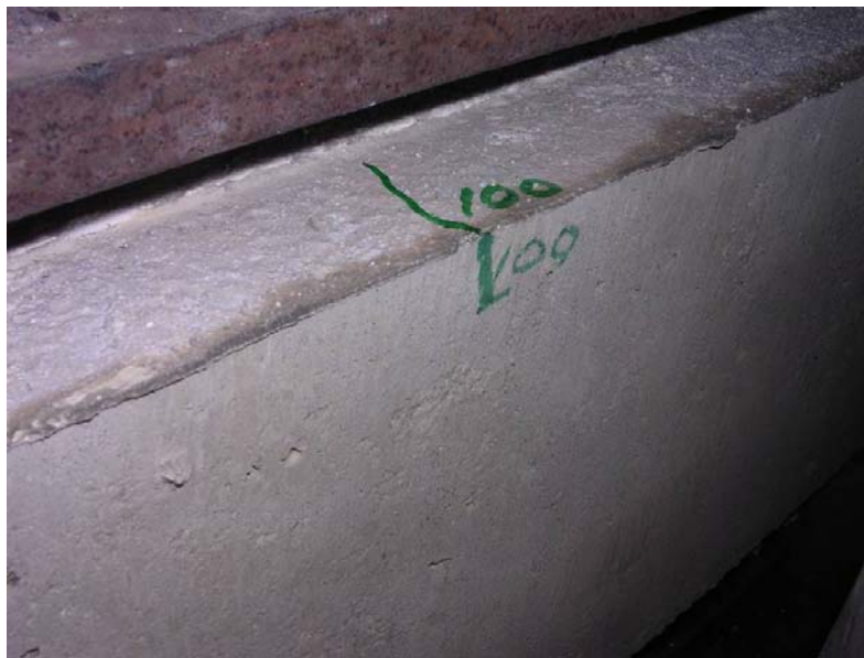
Figure 7.107: Initial Cracking on Concrete Jacket #2 Specimen
