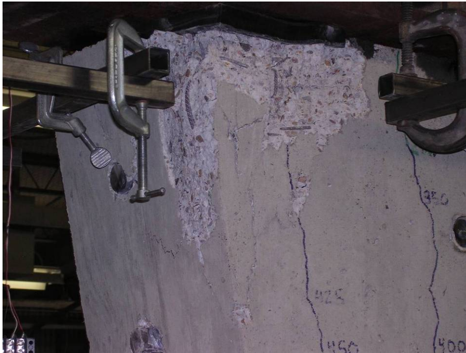
Figure 3.4: Concrete Spalling and Crushing under Heavily Loaded Bearing Pad
